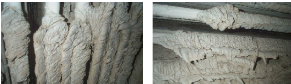
Figure 4–5 Secondary super heater fouling: potassium sulfate (left); potassium chloride (right).
